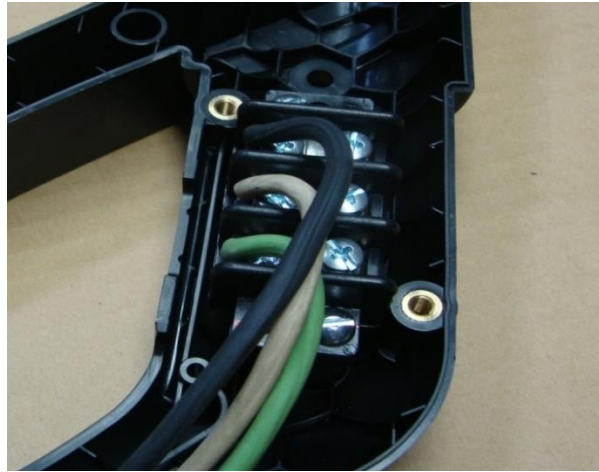
Fig.6-19 Terminal Block Wiring
